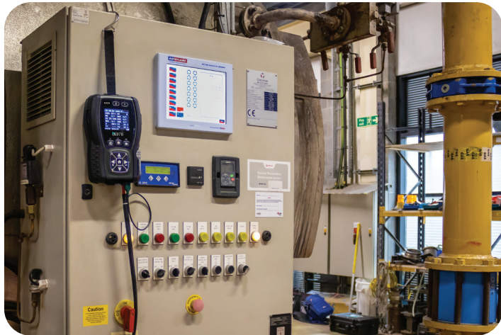
Industrial Boiler Analysis
