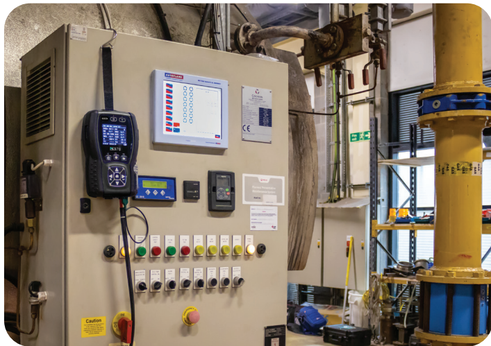
Industrial Boiler Analysis
