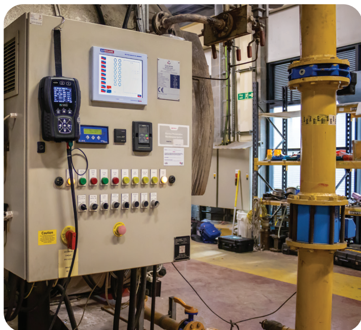
Industrial Boiler Analysis
